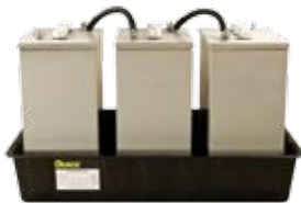
Battery tray with three L16/GC2 batteries 120221
